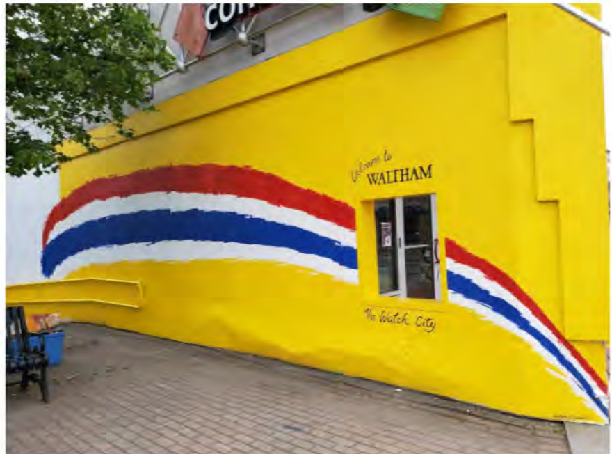
The condemned structure at the 200 block of Moody Street. Mural by Shawn and Donna Laswell. Photo by Chris Wangler. Courtesy of Waltham News Watch.
