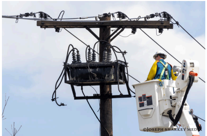
A technician works to repair the blown transformer. Photo courtesy of Joseph Sharkey Media.
