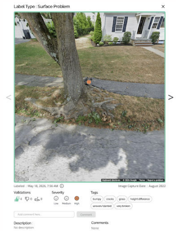
A broken sidewalk identified by the students. Courtesy of Project Sidewalk.
