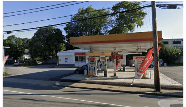
The overhang at this Shell station was damaged by a box truck. Google Street Image.
